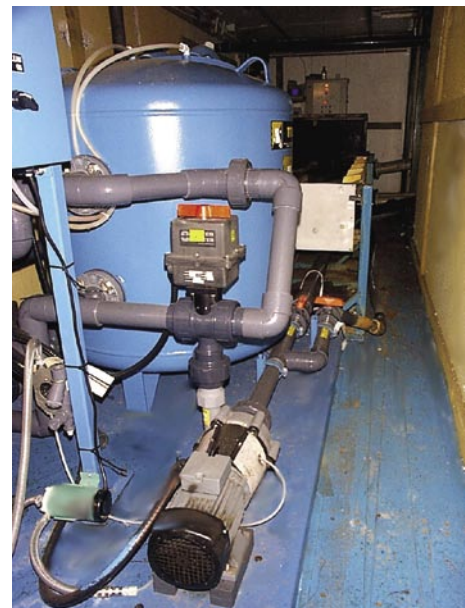
The Recirculation and Backwash Pump, showing Automatic Valves
