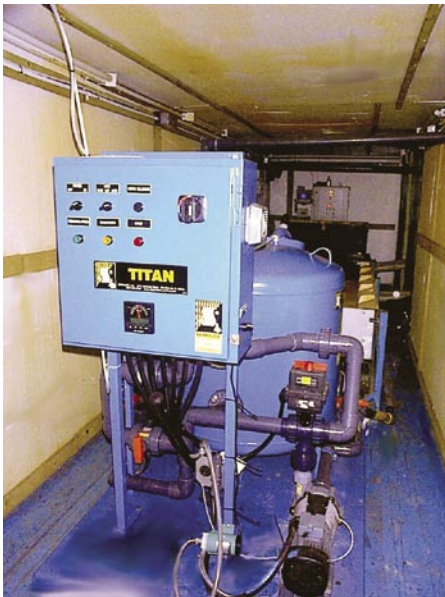
Totally automatic PLC Controlled Titan and BackWash Filter Vessel
