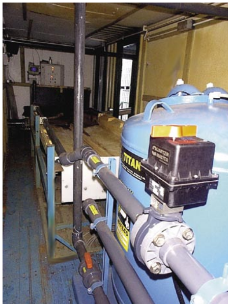
Closed loop return pipework to the central re-circulation tank
