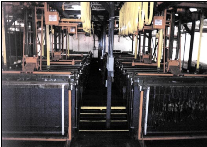
New plating lines installed by IEP as part of their expansion after the fire at the end of 2000.
