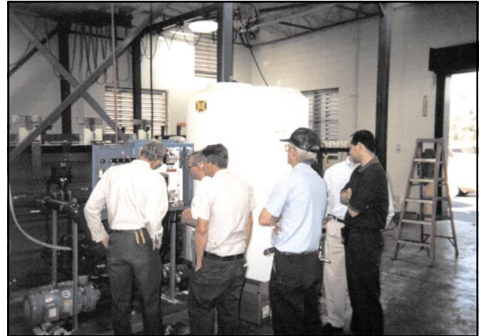
IEP's maintenance staff and shop manager, Scott Curtis (dark shirt) observe a SERFILCO service engineer checking out the automation on one of the TITAN units prior to filter operation.
