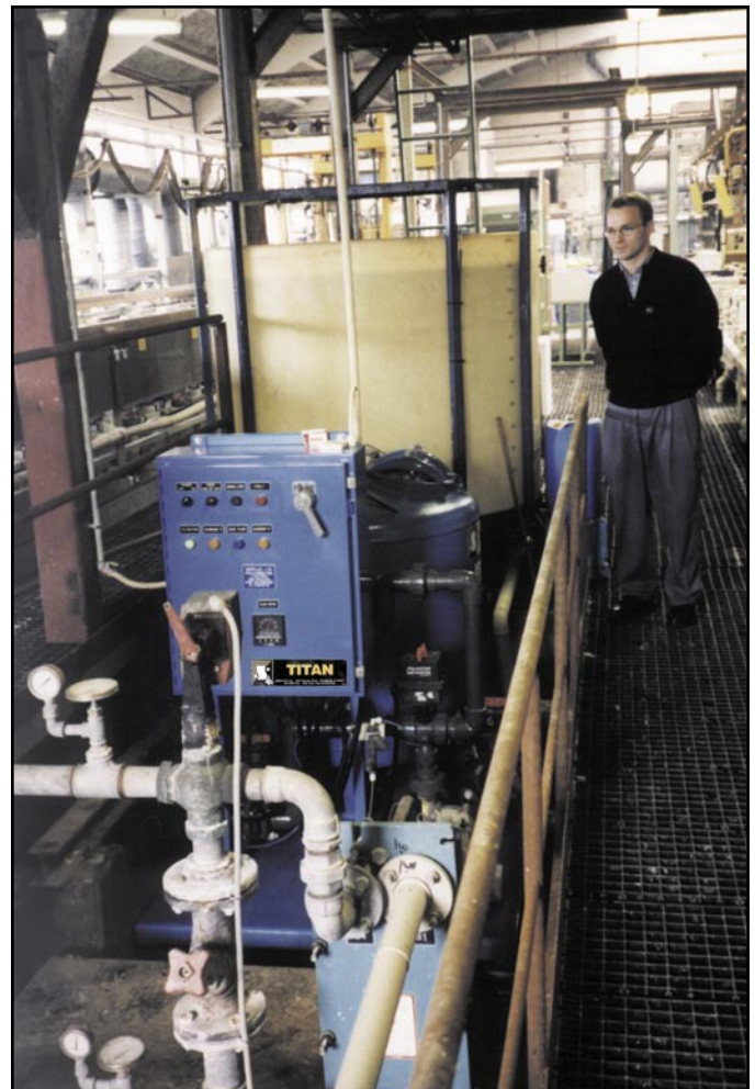
Ib-René Therkildsen, Sectional Engineer - Screw Sector at NKT views the automatically controlled SERFILCO TITAN permanent media filtration system.
